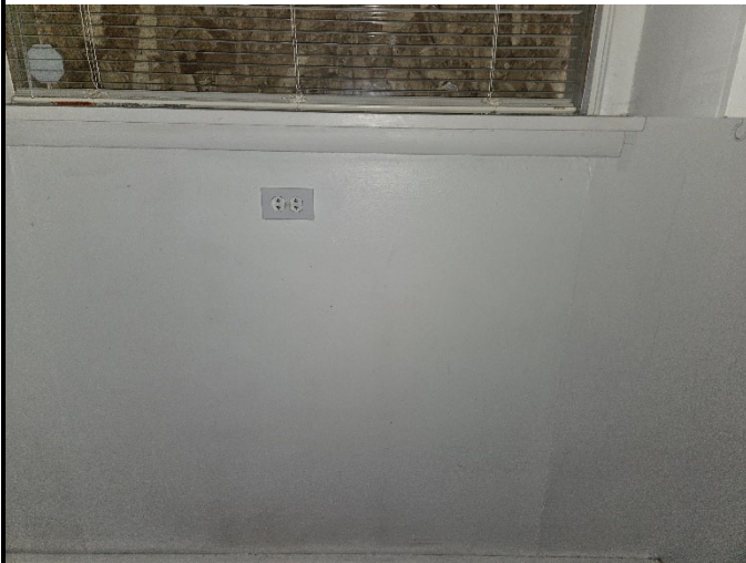
Photo 9. Lead-based paint in hallway, Wall A – LBP28
