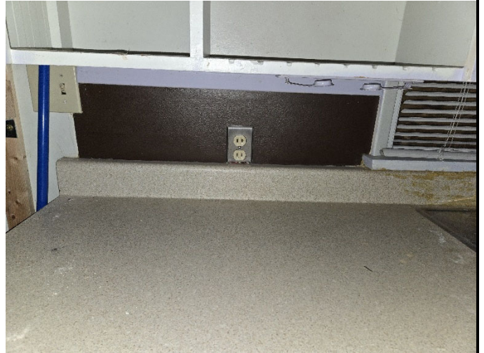
Photo 10. Lead-based paint in kitchen, Wall D – LBP40
