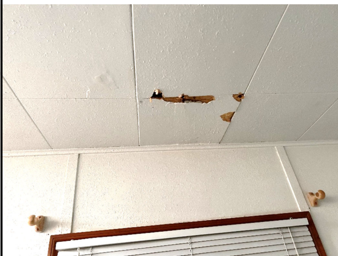
Photo 5. PACBM and PCBs sampling location, ceiling tile in Room 2 – Sample AS05/PCB05
